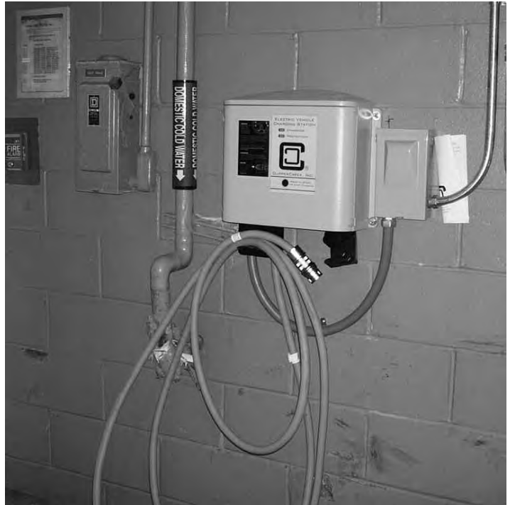
The 220V 32A fast-charging station, with a proprietary connector, fully charges the vehicle in 3-4 hours
